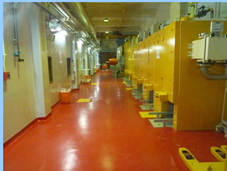
Hot corridor view
